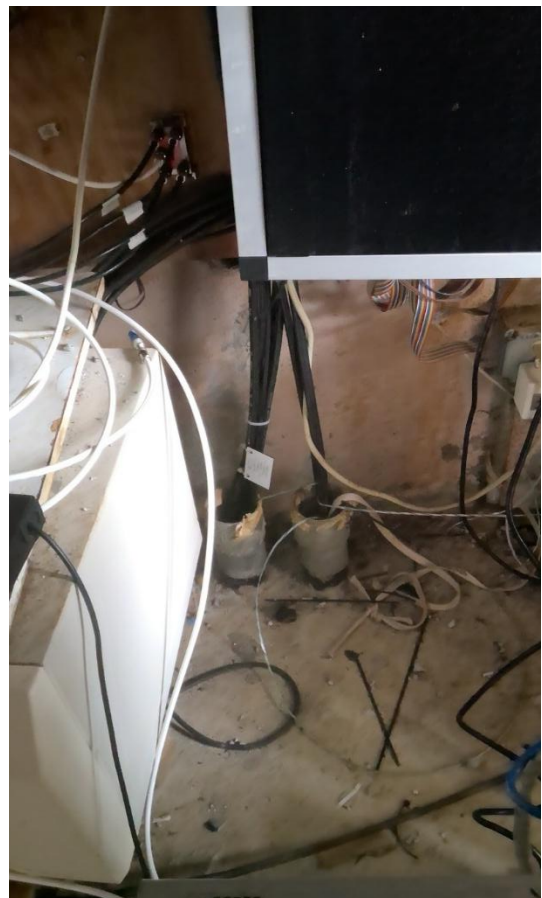
Photo 10 – Conduit pathways connecting to Kaala & Building C
