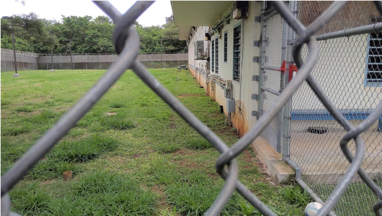
Photo 27 – Exterior pathway penetration into Kaala CCTV room
