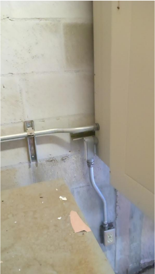
Photo 5 – CCTV cabinet power supply
